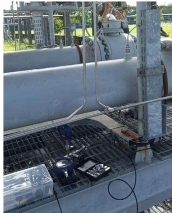
Gambar 4. Validasi Bulanan Metering System
