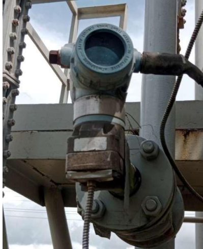
Gambar 4. Level Transmitter 02-LT-050
